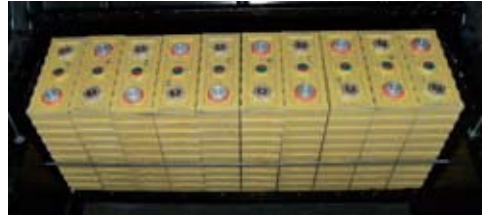
A bank of LiFePo4 batteries
