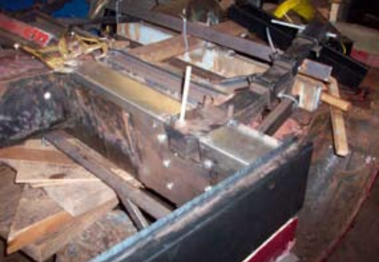
Springs jugged in position along with the new sills and some plate work
