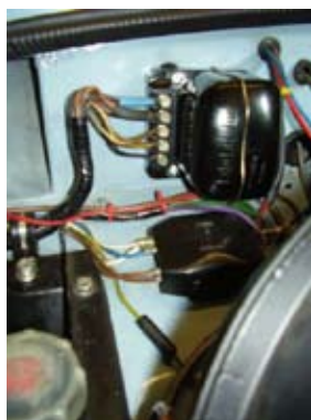
The final wiring set up
