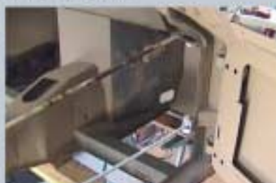
▲ The temporary door brace can be seen here. Other areas to need attention were the boxes of the A-pillars. Again, Dave cut them out and welded in new sections.
