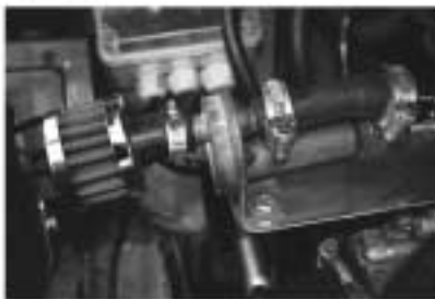
Below right: Relay box keeps things tidy.
