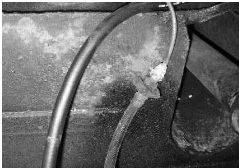
Rusty Hose Connection
